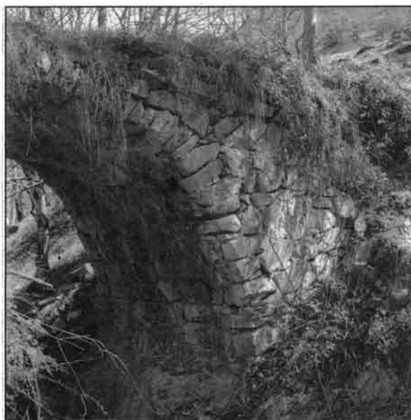
Top. Bridge seen from south and the right bank pylon (XVI-XVII cent)
