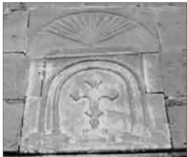
AKANA (AKN). Sourb Hreshtakapetats (Holy Archangels') Church as seen from the west and south-west; a khachkar and a cross relief (17th to 18th cents.) on the southern and western walls of the church
