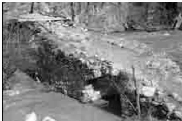
GARNAKER (BARUMSHEN). The remnants of a double-span bridge over the river Shamkor
