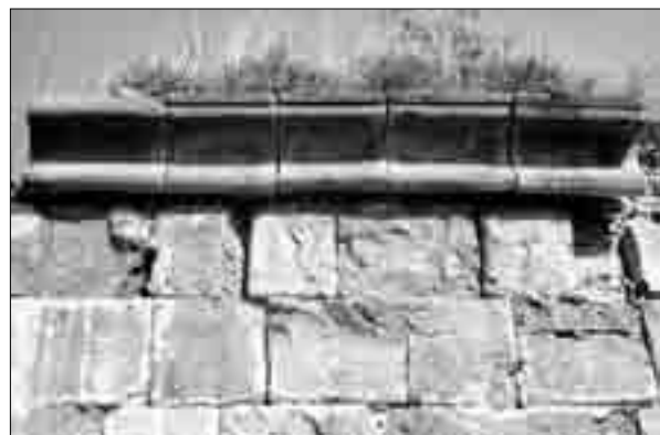
GETASHEN. A partial view of the monastic dwellings; the construction inscription of one of the rooms (1712), and part of the cornice of the southern facade of the church of Yeghnasar Monastery
