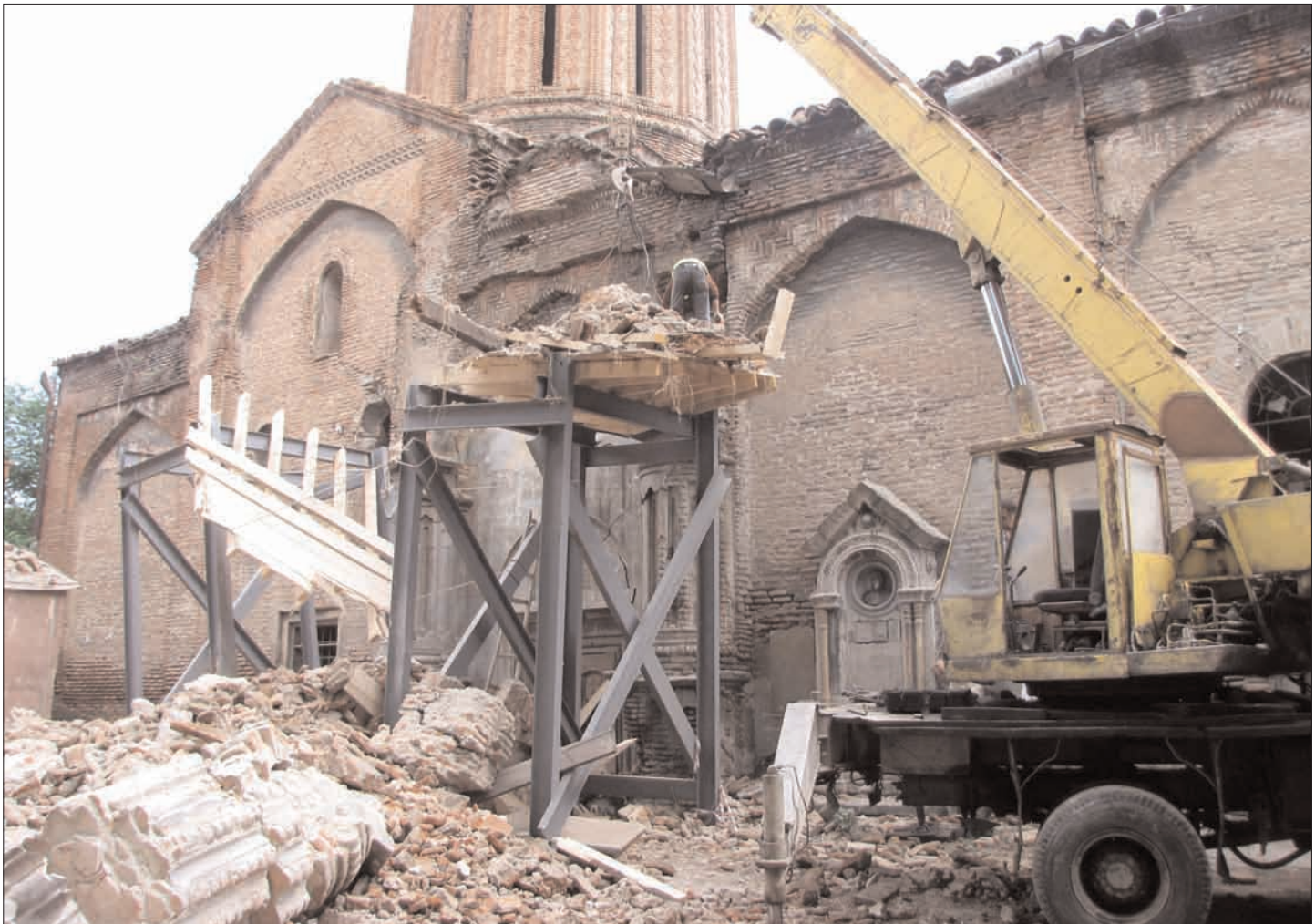
The porch built in front of the northern entrance of Sourb Nshan (Holy Sign) Church as totally destroyed on 14 May as a result of the heavy showers of the preceding days (photo by N. Akopov, 14 May 2012)
