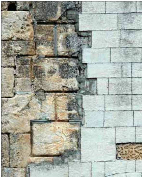
MALABADE. General and partial views of the “restored” bridge
