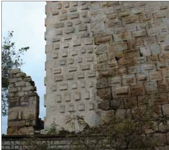
TIGRANAKERT. A partial view of the “restored” ramparts of the castle
