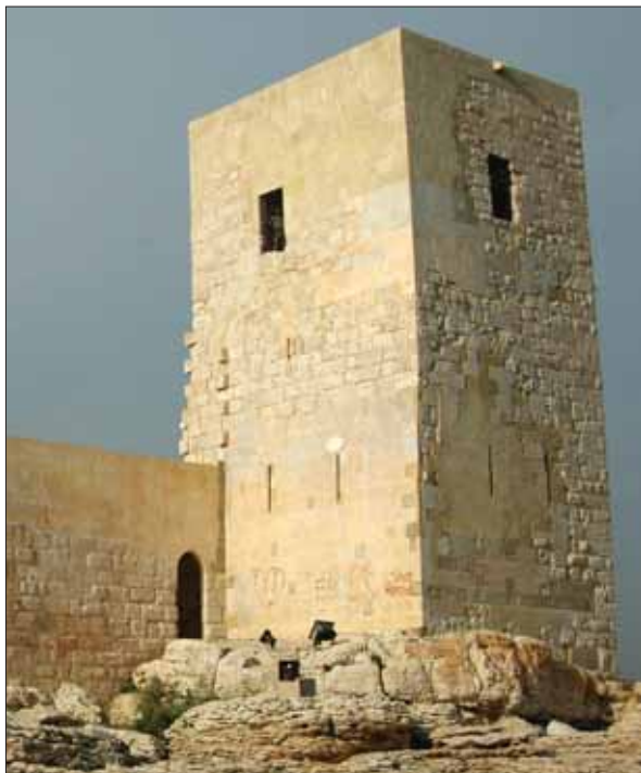
KORIKOS. The eastern tower of the castle before and after its restoration
