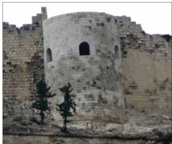
SELEUCIA. One of the restored towers of the castle; partial views of the “restored” fort ramparts
