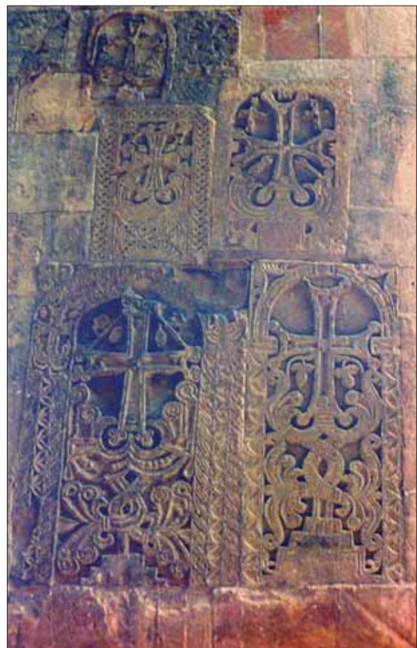
Cross-stones inwardly set in the southern wall of the cathedral during its 13th-century overhaul (photos 2000): they have been amidst ruins since 2005 to 2006, when that part of the wall collapsed.
