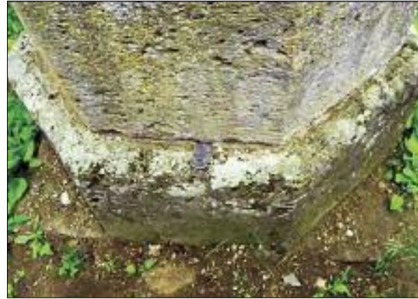
The ruler inserted in the area of contact between the two blocks of the pillar base, 2014
